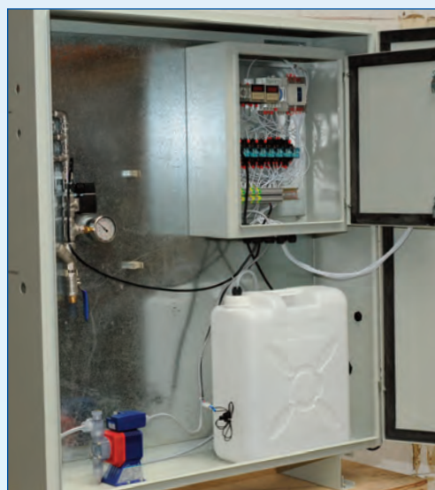
INTERIOR OF AUTOWASH CABINET
